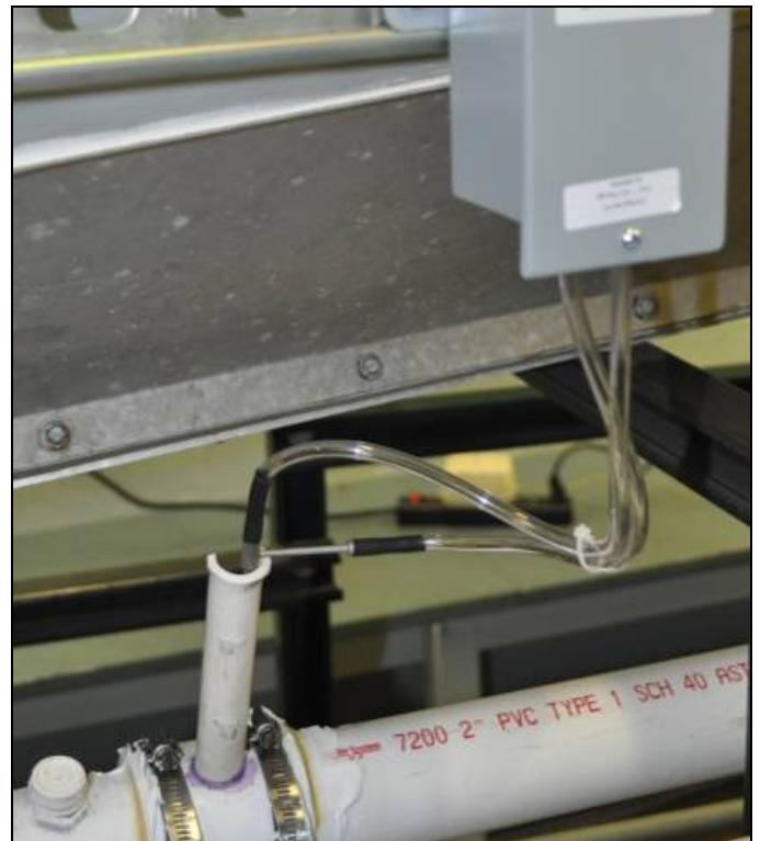
Figure 5. Pilot Tube and Differential Pressure Transducer.
