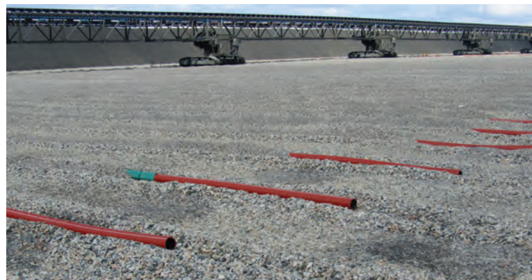
Figure 4 Typical underheap solution collection pipes
